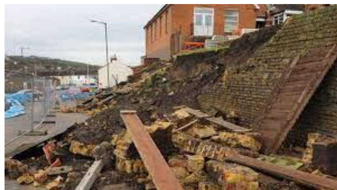
Plate 6 – collapsed boundary wall mid-January 2016 (Kent online, 2023).
